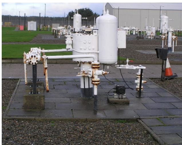
Figure 3: Typical gas-powered Actuator at St Fergus terminal
