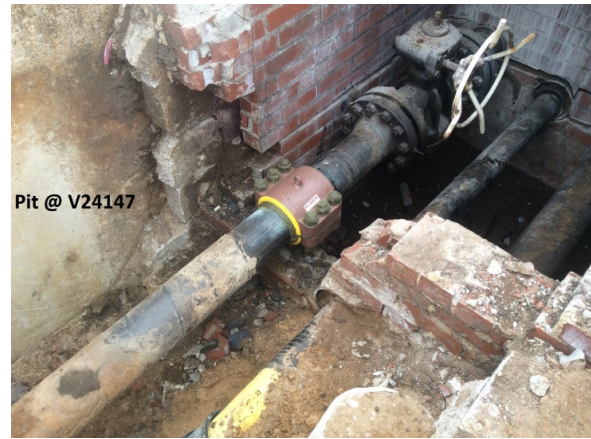
Figure 12: Temporary Plidco Clamp on Actuating pipework at pit wall transition
