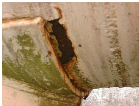
Figure 7: Corrosion under pipe support - a difficult failure to identify
