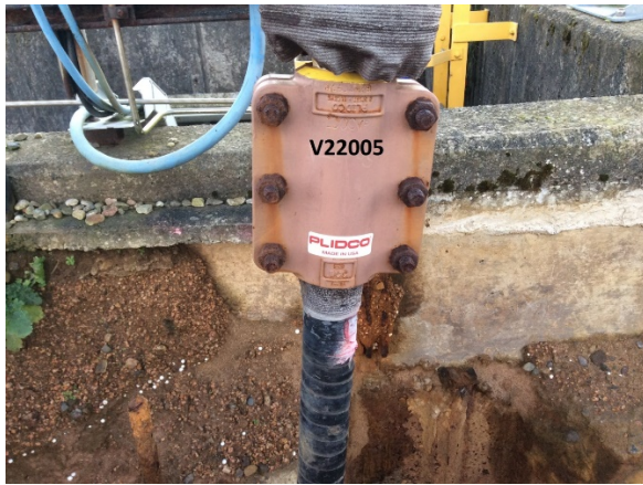
Figure 11: Temporary Plidco Clamp on Actuating pipework riser
